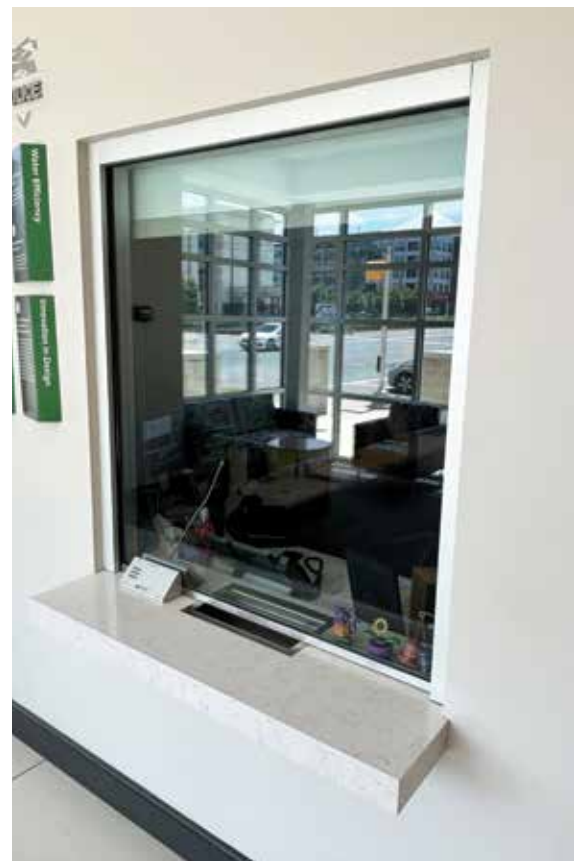
A ballistic-rated USBP transaction window was installed in the reception area to control access into the station and provide for the safe and secure exchange of goods with the public.
